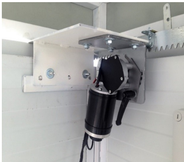
Fig. 3. Detailed installation of motor, clutch, encoder and chain of displacement.
